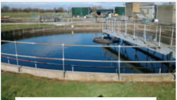
Figure 8. Secondary Clarifier After Trial
