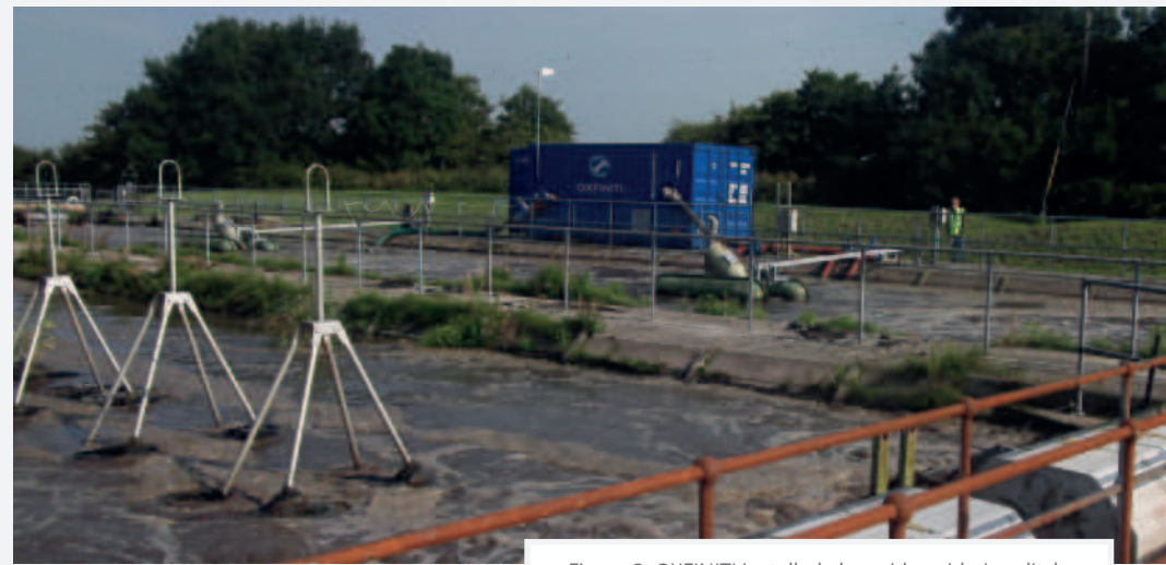
Figure 2. OXFINITI installed alongside oxidation ditch
